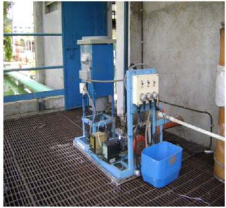
CHLORUN DOSING SYSTEM SIDE VIEW
